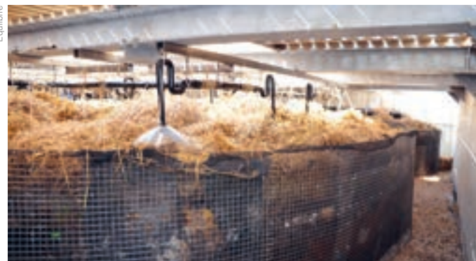
Photo: Vermifilter installation at the housing cooperative, Equilibre, in Geneva, Switzerland. The installation is located underground in the yard of the apartment building and covered by a wooden terrace upon which children play and adults stop to chat.
