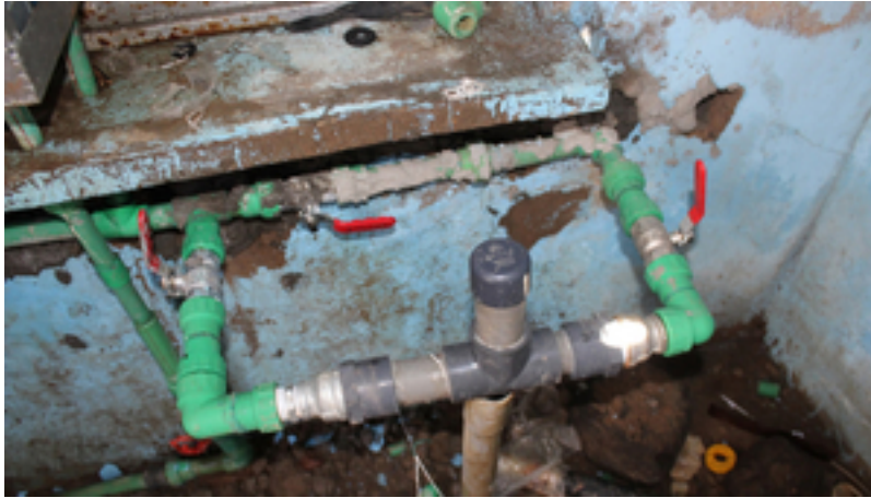
Passive, locally manufactured chlorination system installed in a water kiosk in Kenya. (Photo: Lisa Appavou)
