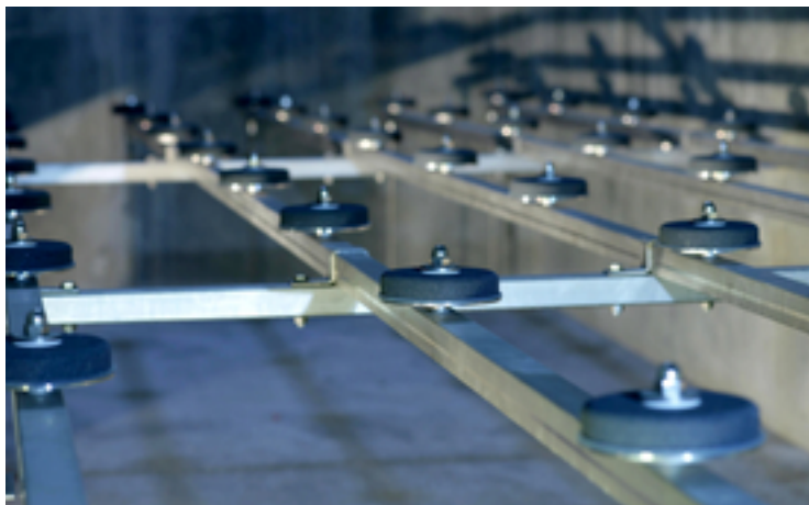
Ozonation is a proven method for removing trace substances from water. In the picture: Ozone diffusers at the Neugut WWTP in Dübendorf. (Photo: Aldo Todaro, Eawag)
