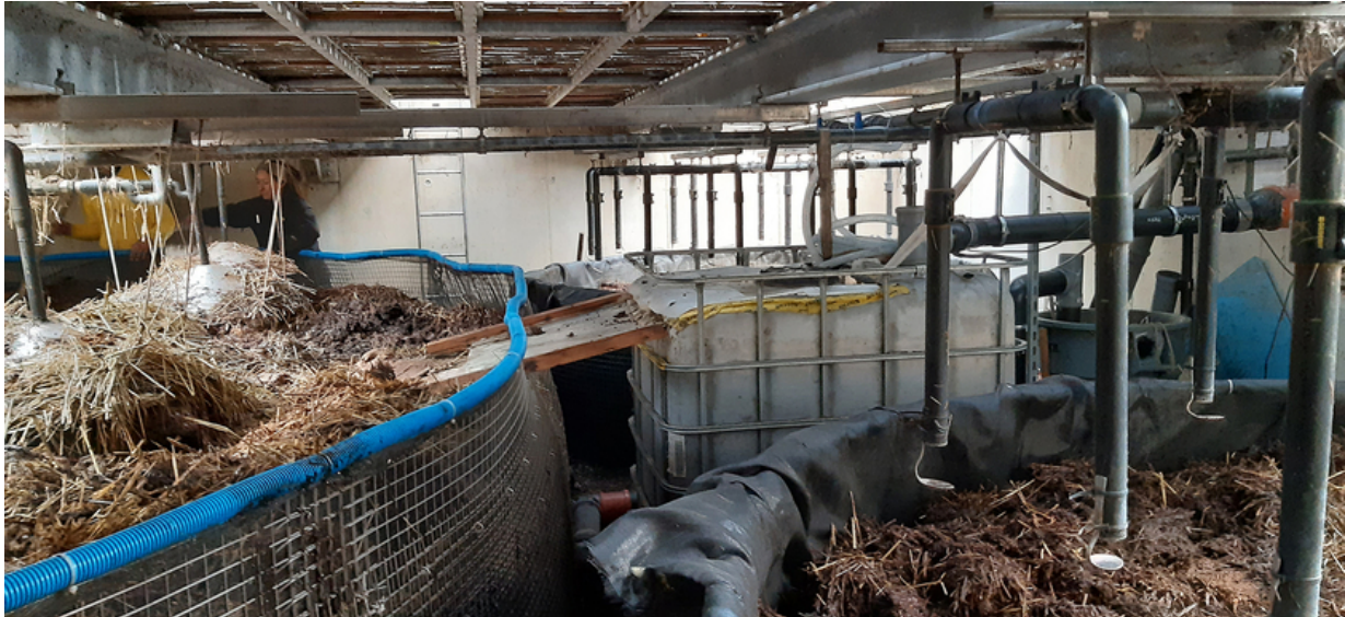
Vermifilter setup at the housing cooperative Equilibre in Geneva (Photo: Eawag, Kayla Coppens).
