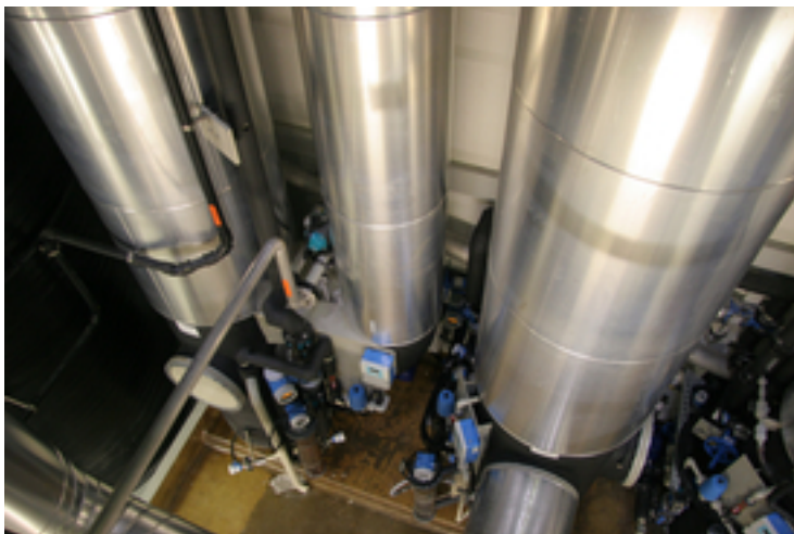
Air-stripping installation for nitrogen recovery at the Opfikon wastewater treatment plant. (Photo: Eawag, Yvonne Lehnhard)
