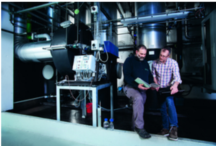
Air-stripping installation for nitrogen recovery at the Opfikon wastewater treatment plant. Photos: Eawag, Peter Schönenberger (left), Eawag, Aldo Todaro (right)
