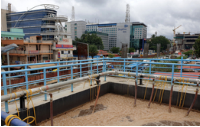
Left: Blackwater treatment system at the new waterfront neighbourhood Mission Rock in San Francisco (Photo: San Francisco Public Utilities Commission)
