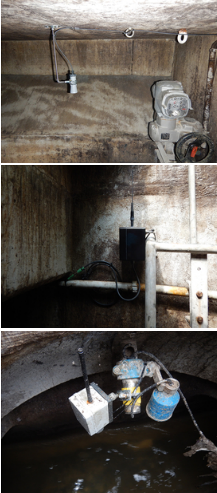
Fig. 2: The wireless sensors transmit spatially and temporally high-resolution measurements of drainage and water levels to the researchers.
