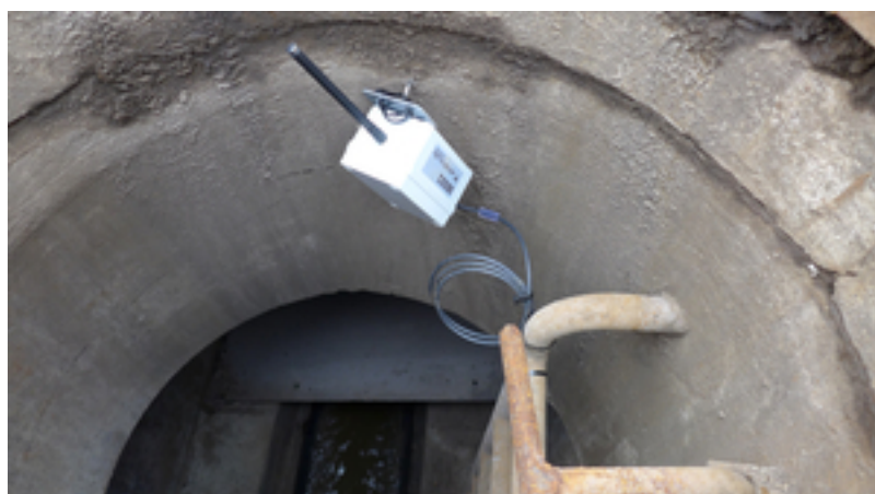
Level sensor with wireless transmission in a sewer (Photo: Frank Blumensaat, Eawag)
