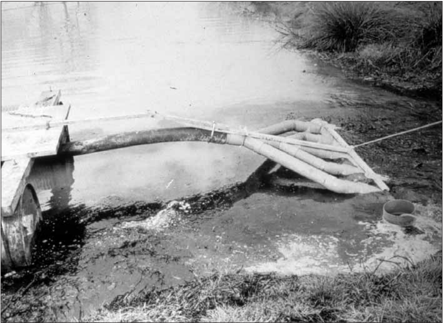
Figure 14.2 Pond Desludging in Northern France using a Raft-mounted Sludge Pump – detail: sludge suction head
