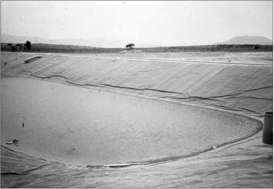
Figure 13.4 Anaerobic Pond Lined with an Impermeable Plastic Membrane
