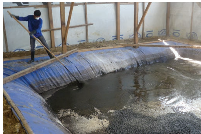
Figure 26. This is a reactor pit in Palo, Leyte, which was first built after Super Typhoon Yolanda. Here, workers stabilize the septage with lime, then transfer it to sand drying beds.
