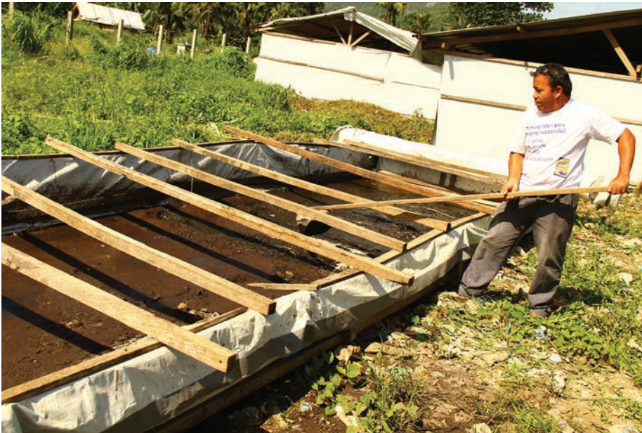
Figure 27. Worker levels stabilized sludge in a makeshift drying bed in an effort to keep biosolids on site in Tacloban City.
