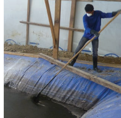
Figure 22. Hand mixing is inefficient and labor intensive. Mechanical mixing with paddles, blowers or pumps is better.
