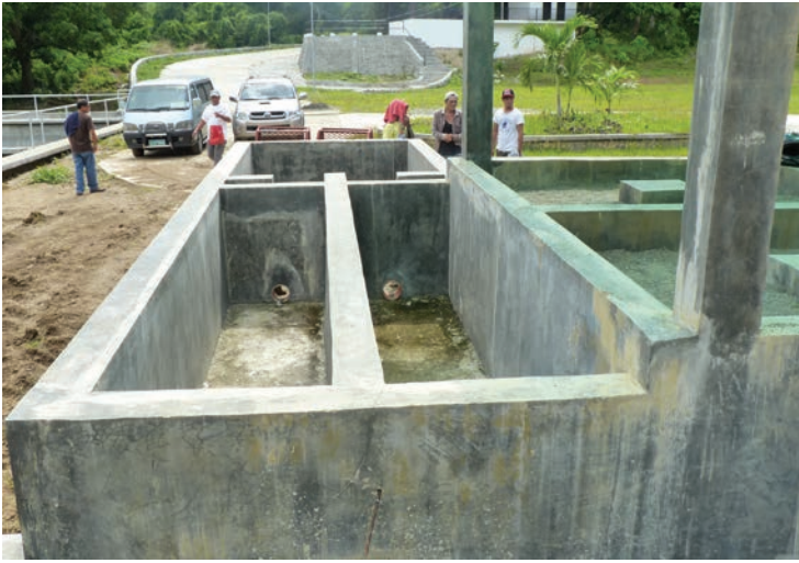
Figure 7. Grit chamber at the San Fernando, La Union septage treatment facility.
