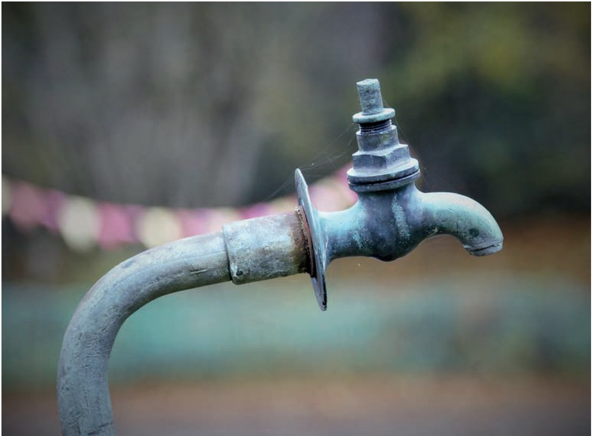
Figure 53: Non-functional water tap (© Jason Allardyce)
