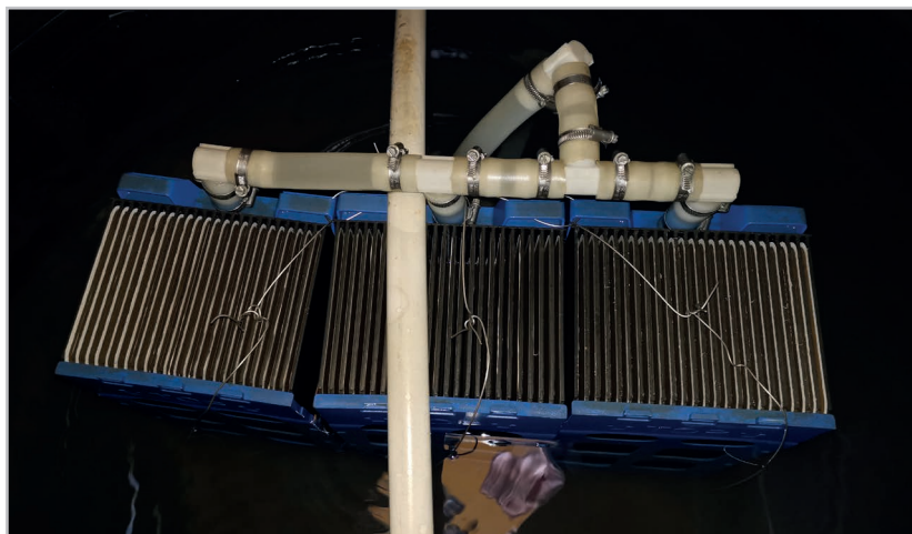
Figure 45: Three TDS-MC-MCXS2 membrane modules installed in Liberia
