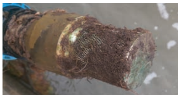
Figure 14: Clogged strainer due to lacking maintenance
