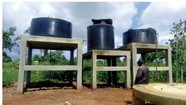
Figure 28: Fundaments of a three tank set-up
