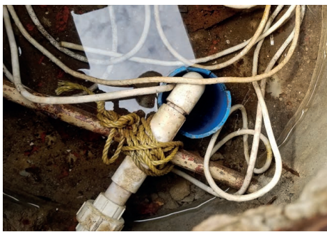
Figure 41: Groundwater well with plastic coat (blue)
