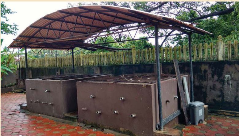
Photo 7.8c Decentralized Composting Units in Panaji, India
