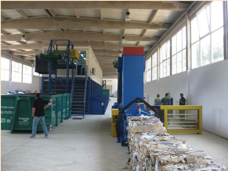
Photo 3.3 Recycling Plant in Bosnia and Herzegovina
