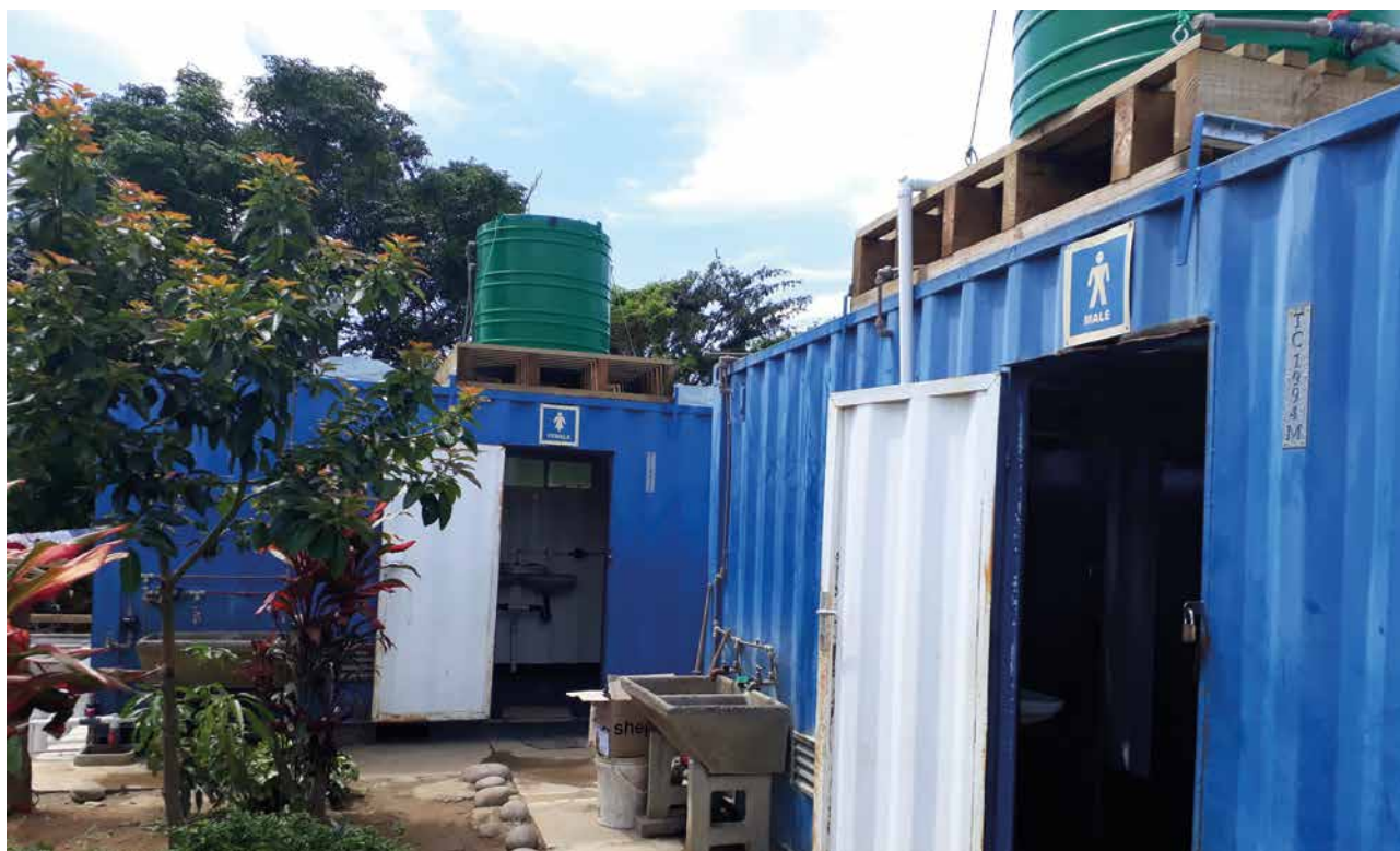
Figure 6: Community toilets in Durban, South Africa.
