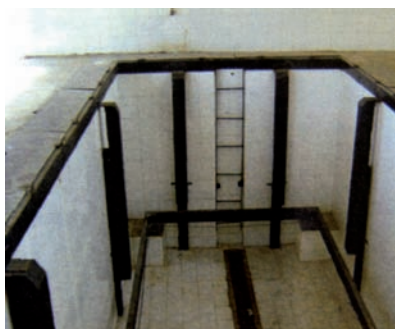
d) Pit for receiving container; note tiled surfaces, drain and weigh cells in corners
