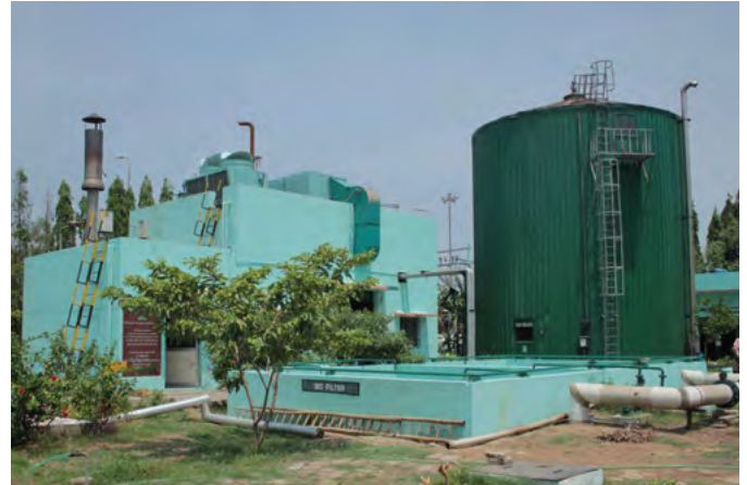
Biomethanation plant at Koyambedu Market with a processing capacity of 30 MT
