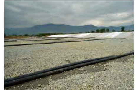
The underground drainage system for leachate collection
