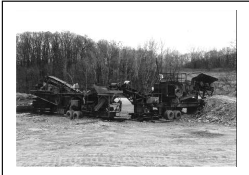
Figure 8. Equipment used to grind building foundation materials for future use on the installation.
