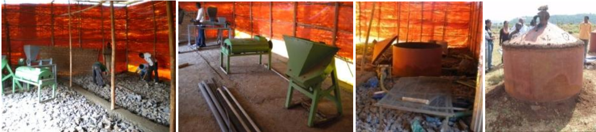
Figure 13: Shed for charcoal briquetting in BD, left to right: preparing the footing for the machines; molding machines, mixer, hammer mill; kiln in shed; kiln during first try-out
