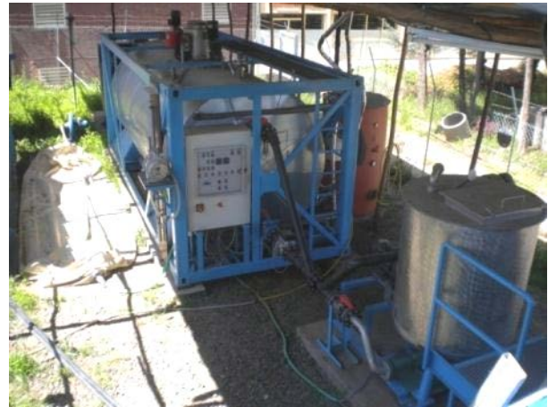
Figure 37: IGNIS pilot biogas plant in Addis Ababa
