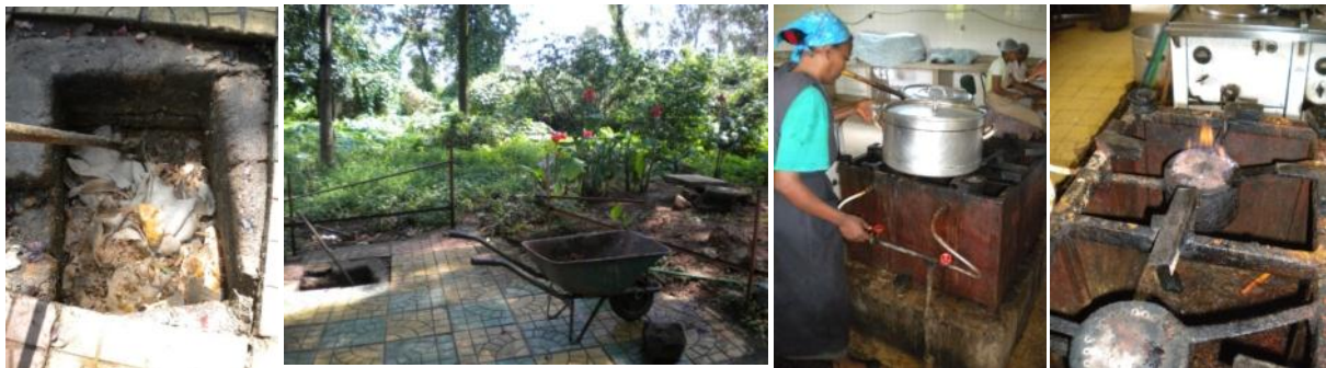
Figure 36: Felege Hiwot hospital: Inlet with kitchen waste, underground AD system, biogas stove, biogas flame (left to right)
