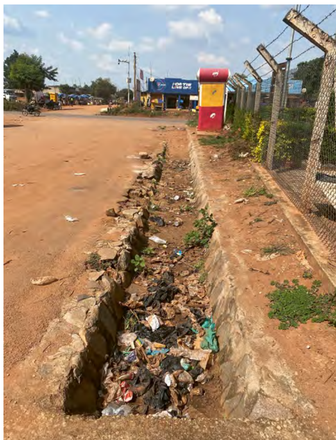
Photo: Solid waste obstructing drainage channels.
