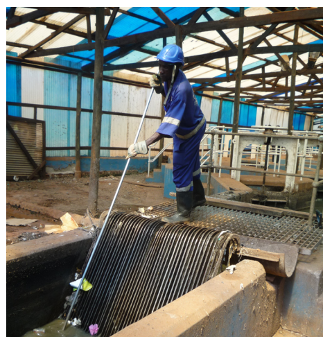
Figure 10: A treatment plant operator removing solid waste from a bar screen with a rake (source: Eawag).
