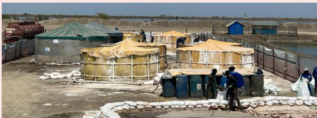
Photo: The lime treatment facility in Bentiu, South Sudan
