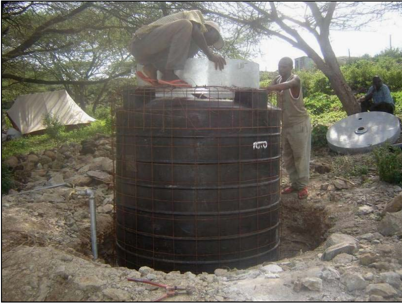
Figure 6-1: Remote community filter under construction. The concrete walling will protect the PVC tank from damage.
